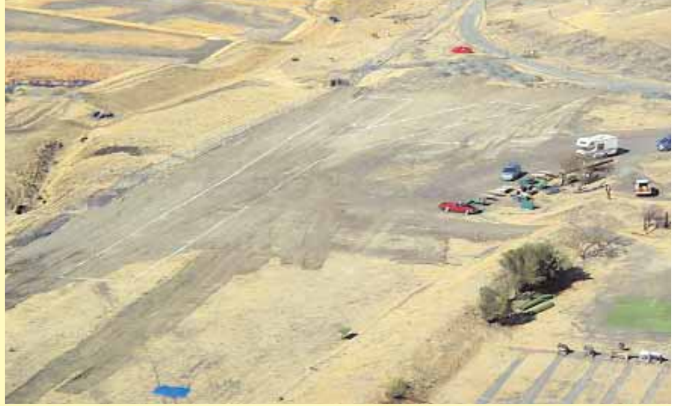
The DVRC site as construction progresses. The members put in a lot of "sweat equity," but the results were certainly worth it! Gallegos photo.
